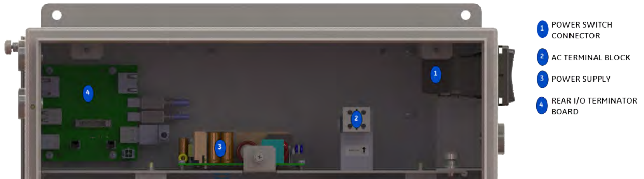
Figure 43: Electronics Enclosure (Top Shelf) — Sievers M5310 C On-Line TOC Analyzer
