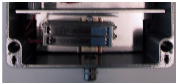
Figure 15. Two dual channel STAHL INTRINSPAK 9002/77-093-300-001 Zener barriers in junction box
