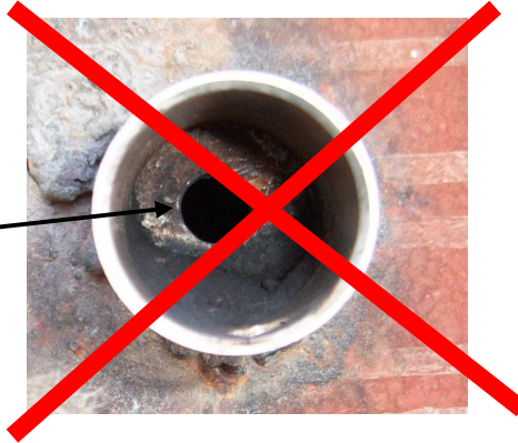
Figure 3b. Wrong socket installation, THE DIAMETER OF THE HOLE MUST BE MINIMUM 38 MM
